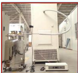
LN 2 /CO 2 backup system
